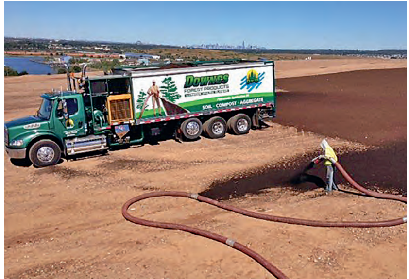
Applying compost mixed with plant seeds to control erosion at Freshkills Park in Staten Island.
